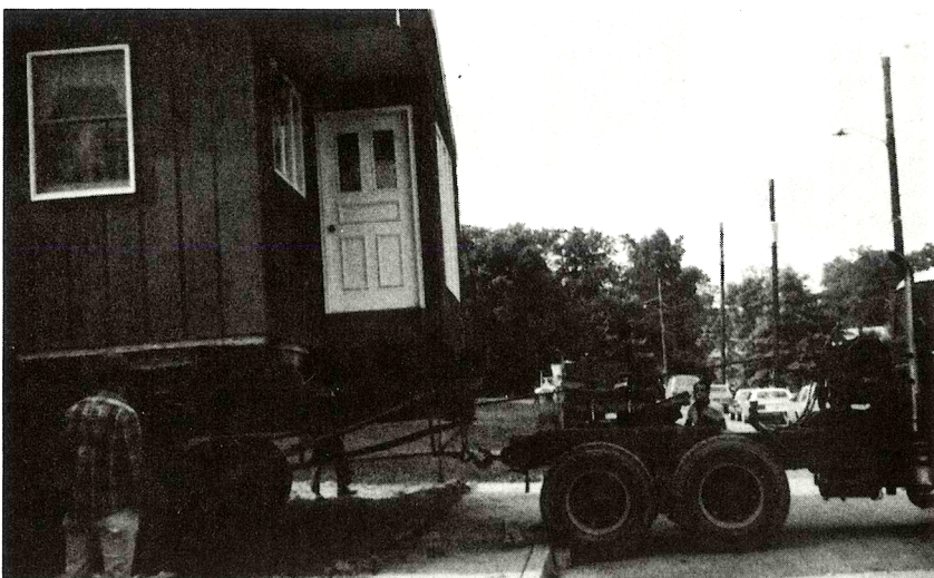
With connections to the truck completed, the journey to the new site begins.
