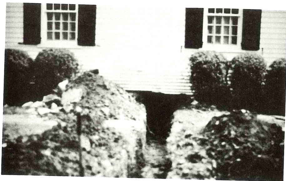
Trenches were dug below the home to allow lifting beams to be placed in position.
