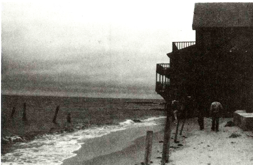
FIGURE 3-22a. This elevated structure was moved from its former piling foundation (on the left) to its present piling foundation because of coastal erosion.
