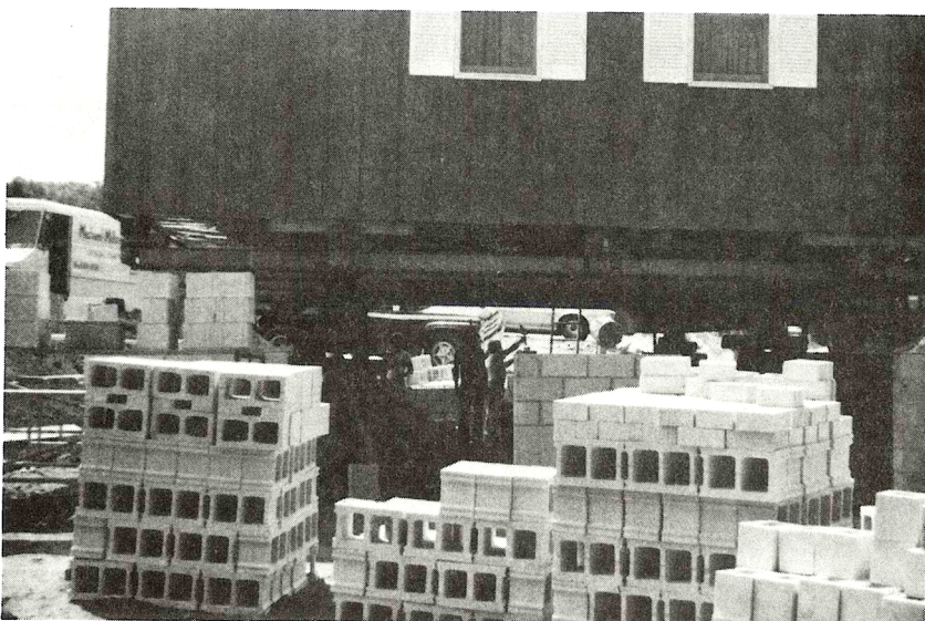
With support cribbing in place, materials for completion of the foundation are readied.
