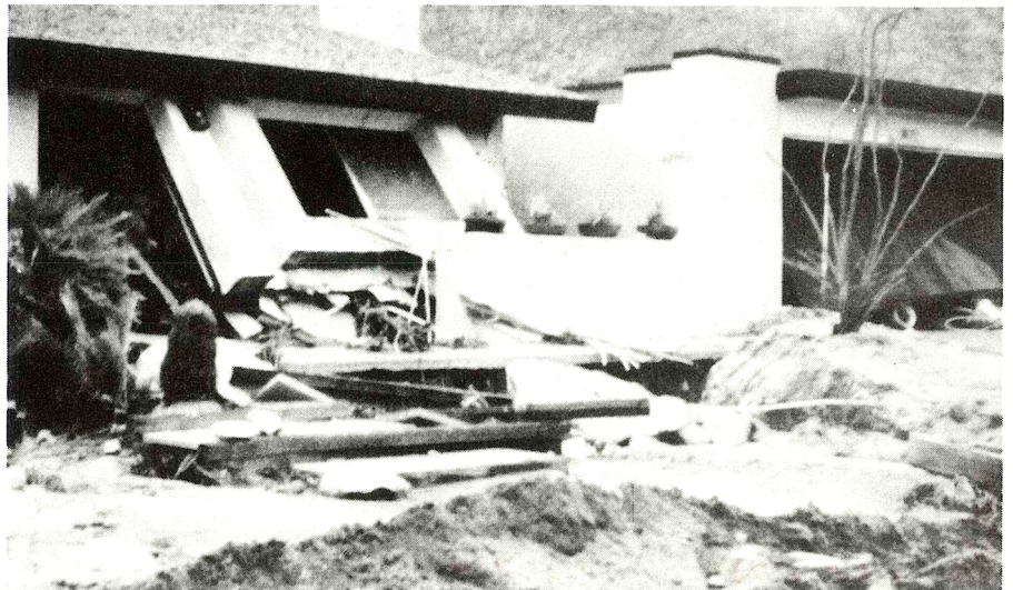
FIGURE 10-3. Due to high velocities and accompanying debris, alluvial fan flooding can demolish a structure.
